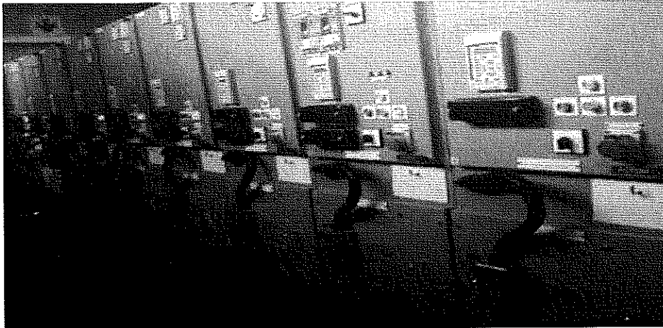
Bela Bela Sub Station
